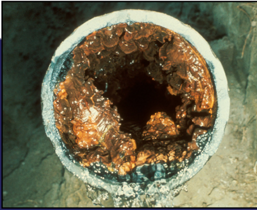
Highly Tuberculated Distribution Line
